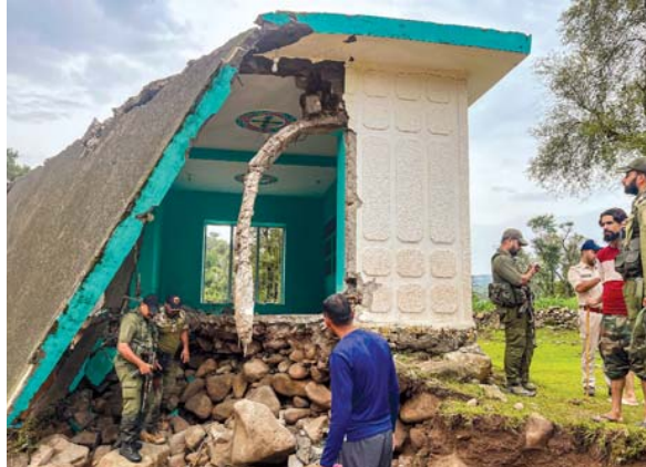
Police inspecting the damage to a mosque after heavy rains and flash floods, in the Mendhar area of Poonch district
